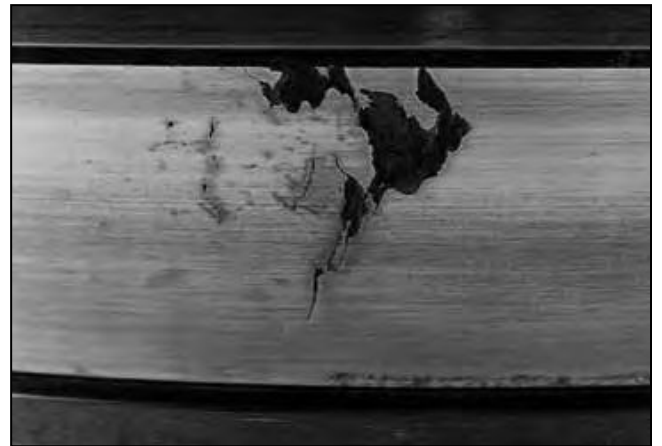
Fig. 170. Point surface origin spalling (PSO).
